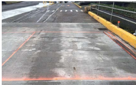
Picture 2. Westbound lane repair area. The drain is located 50' from the fishway.
