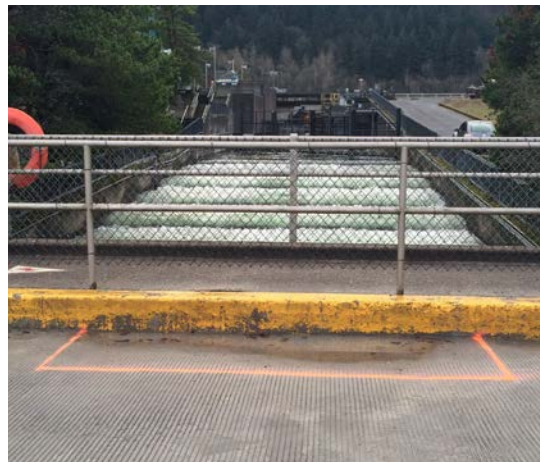
Picture 4. Low spot in the center of the bridge.
