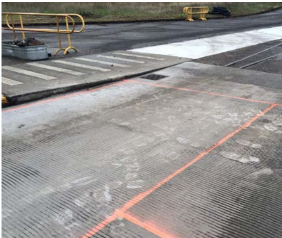
Picture 3. Eastbound lane repair area. The drain is located 50' from the fishway.
